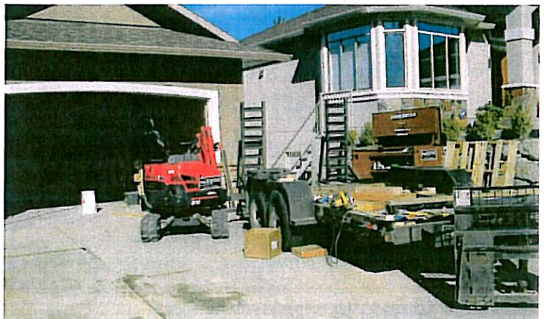
Foundation settlements are difficult to repair
